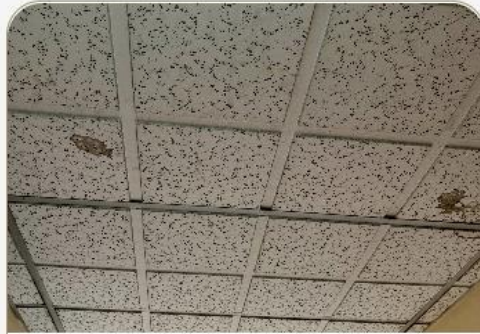
Suspended ceiling & tiles
